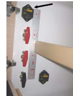
WINDLASS CIRCUIT BREAKER 100A (PORT AFT CABIN)
