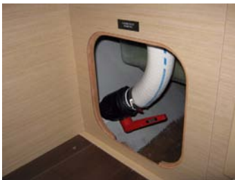
Valve - Drainage to sea (Landmark 1)
