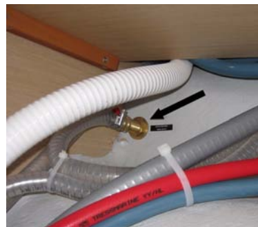
1. Drainage - Refrigeration unit
