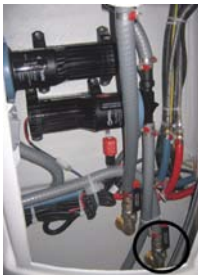
Seawater inlet WC (Landmark 6)
