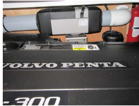
Heater Location: Engine compartment
