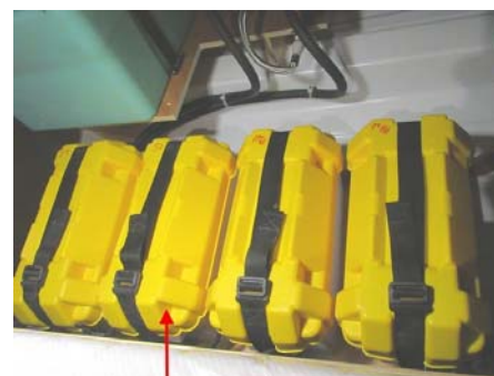
Spare service batteries: 115A
