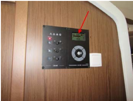
Voltmeter Location: Passageway
