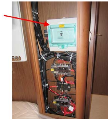
Ref 3: Breaker (Operation)
