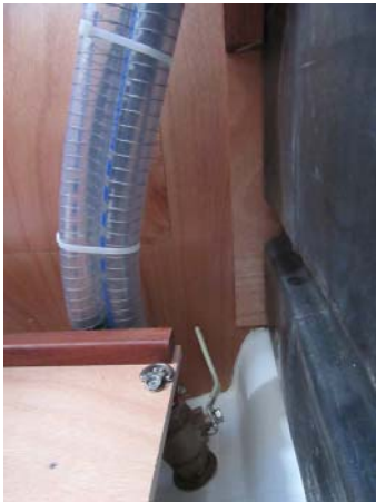
Sea water intake
