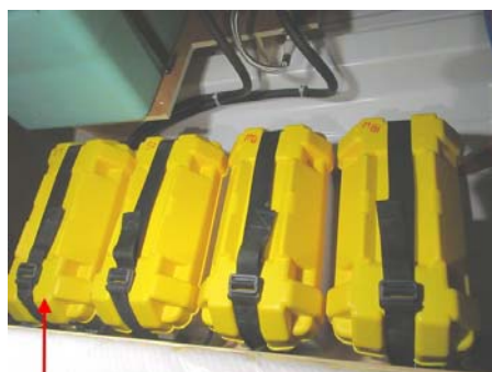
Service batteries: 115A
