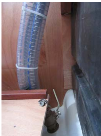
Engine water intake valve: Location: Cockpit locker
