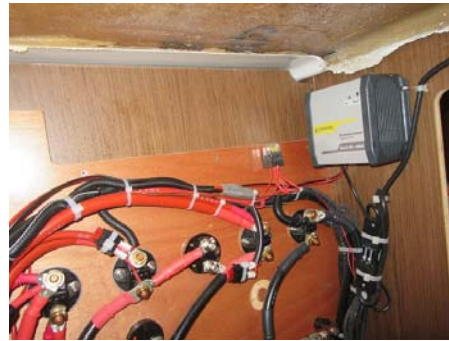
Inverter Location: Aft cabin
