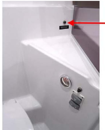
The shower pump control
